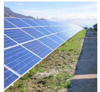
PROVINCE OF SALERNO (ITALY) PHOTOVOLTAIC PLANT 24 MWp
