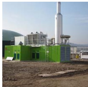
PROVINCE OF MACERATA (ITALY) BIOGAS PLANT 1 MWe
