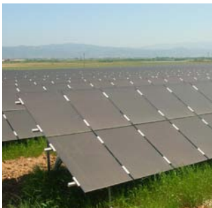
GREECE PHOTOVOLTAIC PLANTS 28,8 MWp
